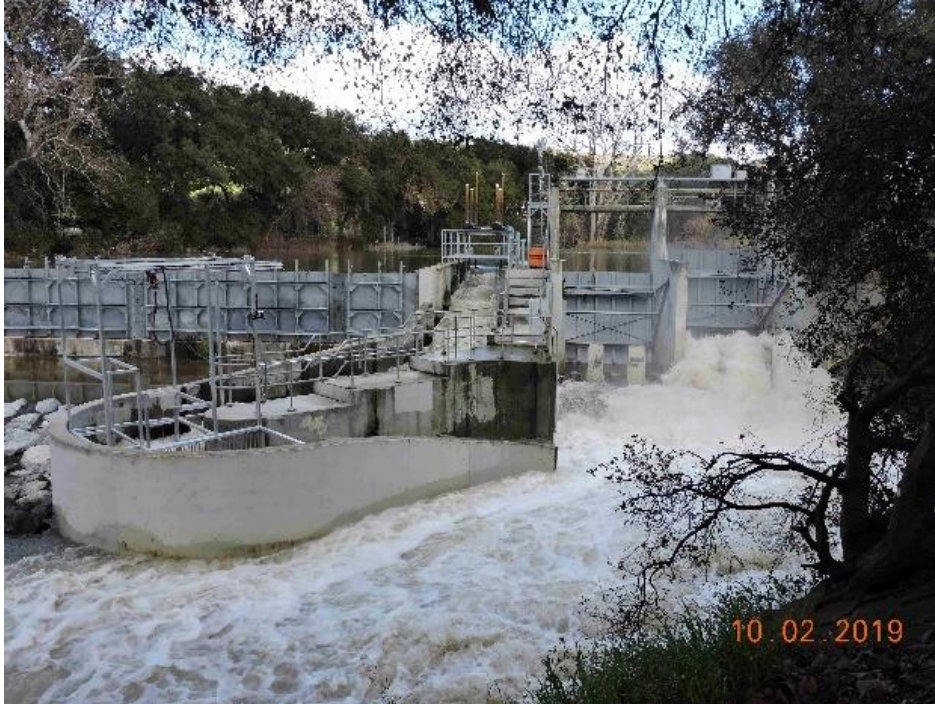
Photo 1. Metcalf Dam on 10 February 2019 at a flow of about 500-600 cfs, due to high releases from Anderson Reservoir to comply with seismic restrictions. One of the radial gates was partially opened to lower the pond water level and prevent overtopping of the dam.
