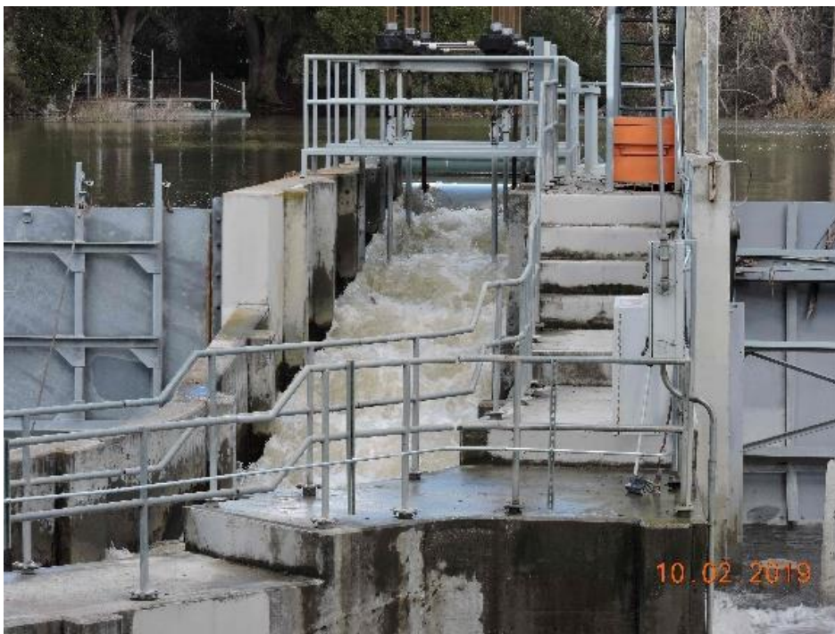
Photo 2. The fish ladder at Metcalf Dam on 10 February 2019. Despite turbulence in the ladder, it was probably passable by adult steelhead (if they successfully located the ladder in the high flows).
