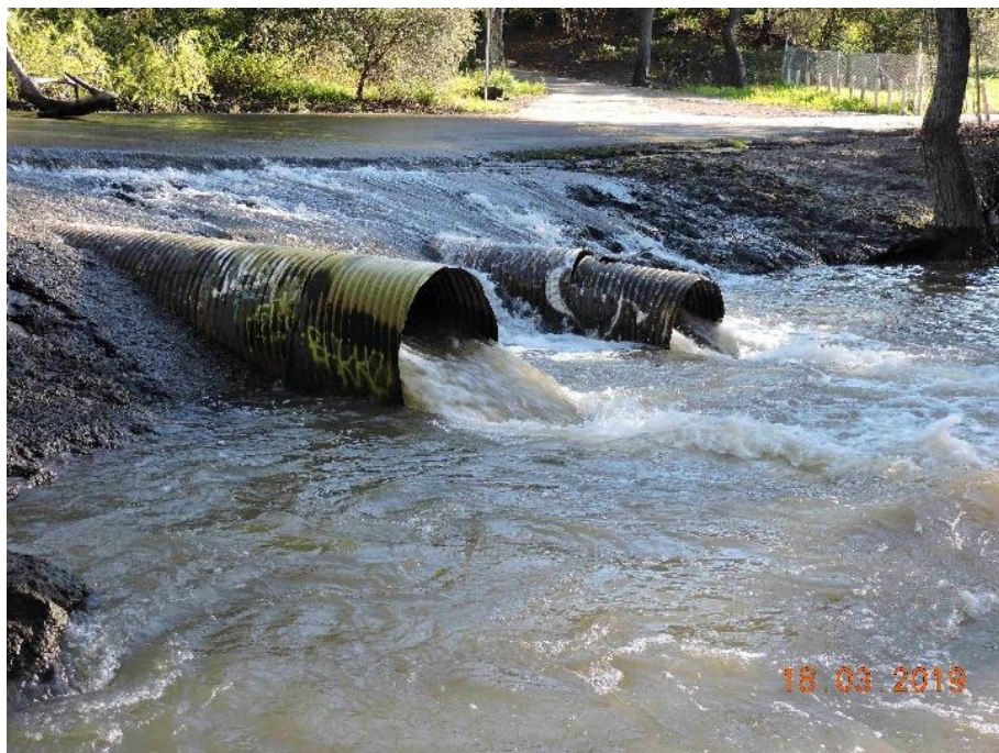
Photo 7. Singleton Road crossing at a dropping stream flow of about 140 cfs on 18 March 2019. High velocity in the culverts and the shallow flow over the apron probably prevented adult steelhead upstream passage.
