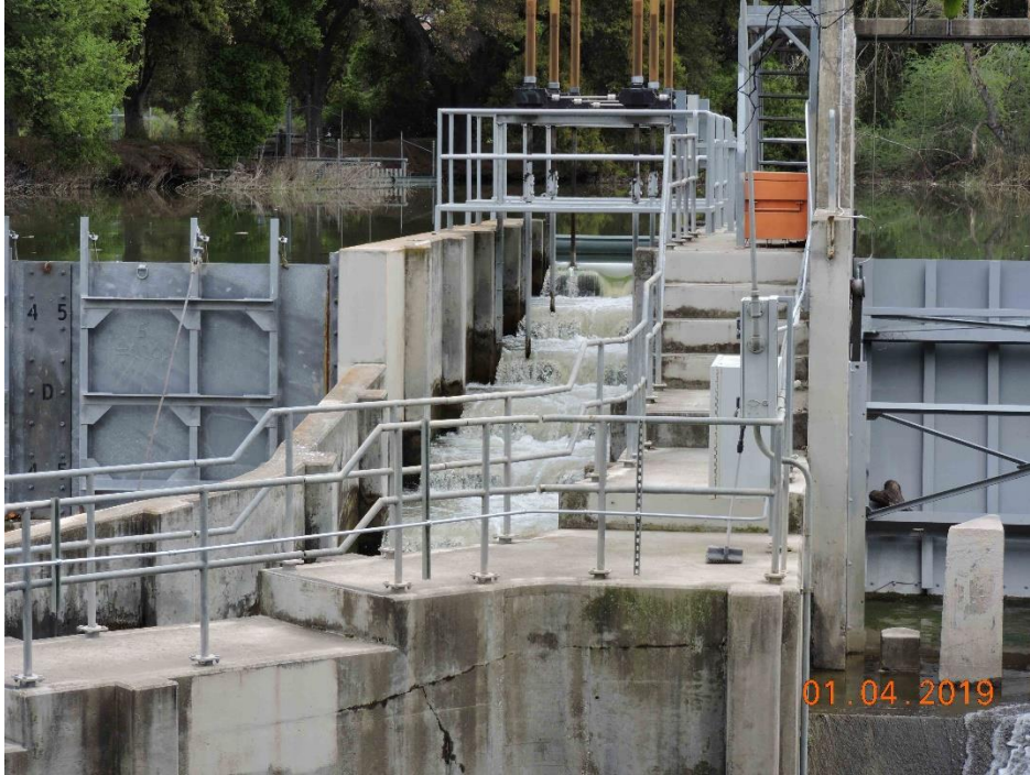
Photo 3. Metcalf Dam fish ladder on 1 April 2019, with radial gate partially open and easy passage in the fish ladder; combined flow below the dam was 54 cfs.
